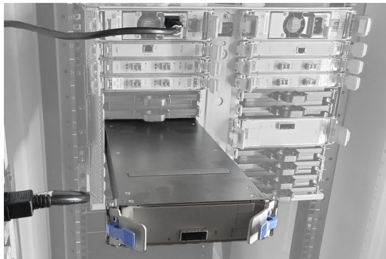
Figure 10: Example Frame Cable Routing Ensuring Serviceability
