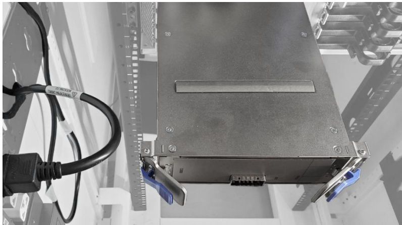
Figure 9: Example Frame Cable Routing Ensuring Serviceability
