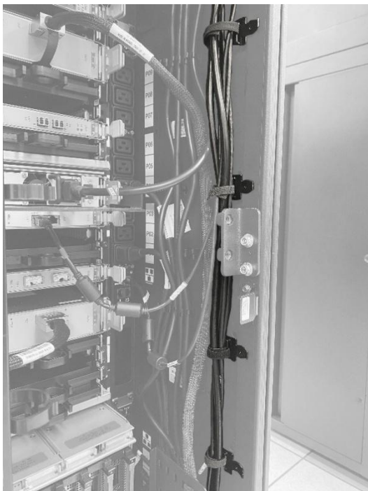
Figure 27: Routing of Excess Power Jumper Cable Slack Using Ethernet Clips
