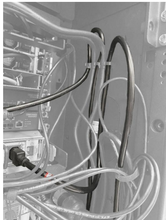
Figure 28: Routing of Excess Power Jumper Cable Slack in Loops Using Clips
