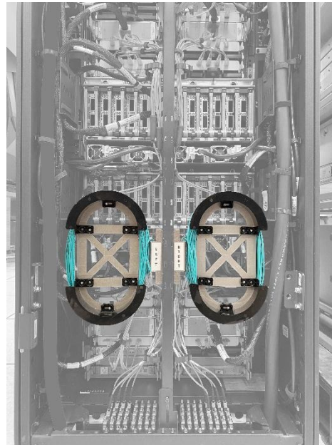
Figure 42: FICON Cabling Spools in their Regular Positions
