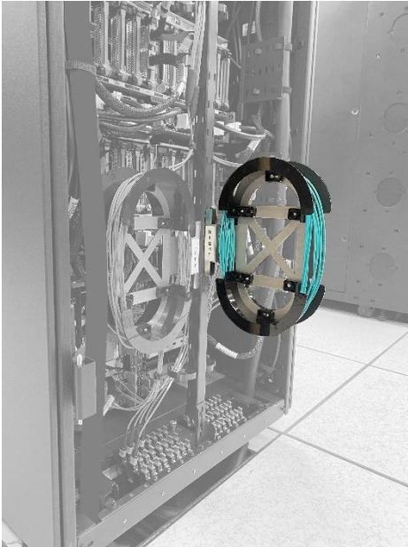
Figure 41: FICON Cabling Spool in its Service Position
