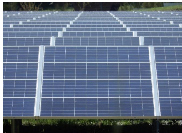
Solar installation at IBM Vaux-sur-Sûre Data Center
