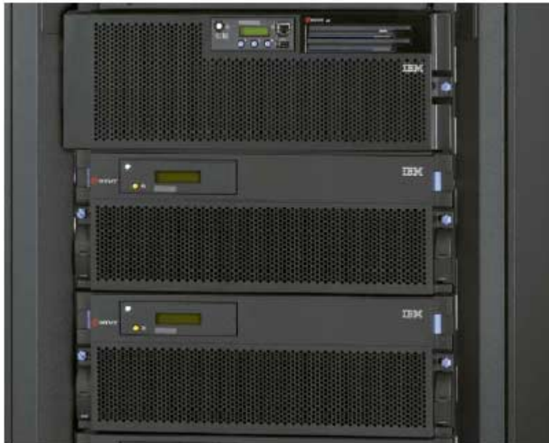
IBM @server p5 570 in rack con I/O drawer
