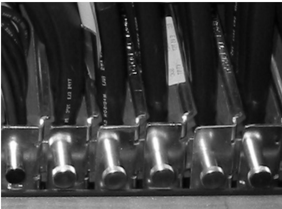
Figure 37. Cable management bracket with cables installed
